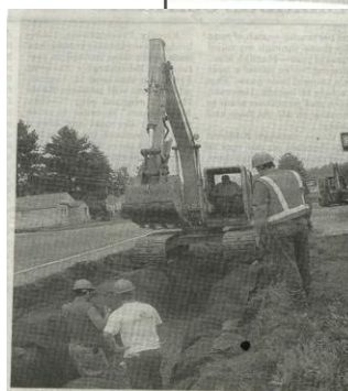
Work is currently being done to implement the Wilkins Ravine-North End Commercial District stormwater cleanup plan. These projects have been funded by grants from the state Agency of Natural Resources under Section 319 or Section 1045 of the Federal Clean Water Act. The federal funds were matched with local funds or resources from the Country Home Center, Pete's Repair and the Town of Morristown. Here the Morristown Highway and Street Department install the stormwater infiltration gallery in front of Menard's Agway and Pete's Repair. Dave Holsington is operating equipment loaned by Pete's Repair. Jim Pease photo
